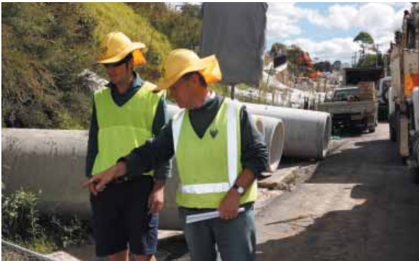
RTA staff carrying out an OHS inspection on the Great Western Highway.
