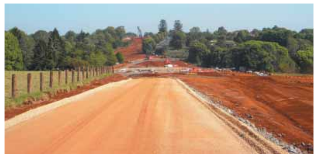
Construction works at the Alstonville Bypass, expected to be completed in late 2010.
