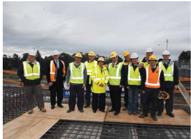
Former Premier Morris Iemma, Dianne Beamer and the construction team during an inspection of the works on the $15 million Mamre Road bridge over the M4.
